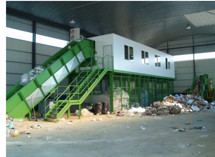
SOLID WASTE TREATMENT Sorting Installation
