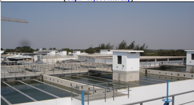
WTP - Maputo (Cap.: 240,000 m 3 /day)
